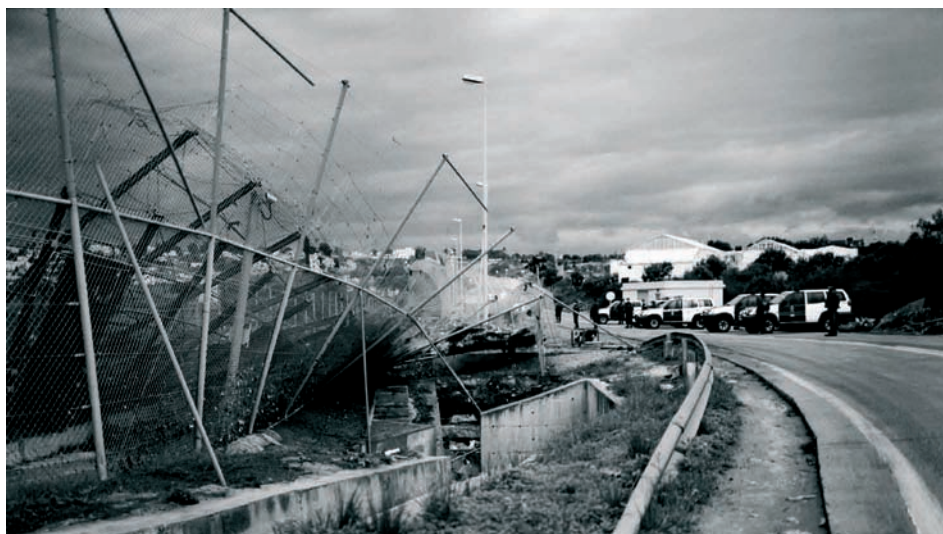
La valla-November 2008, heavy rain has destroyed groundwork of the fence, Melilla Spain, 2008
