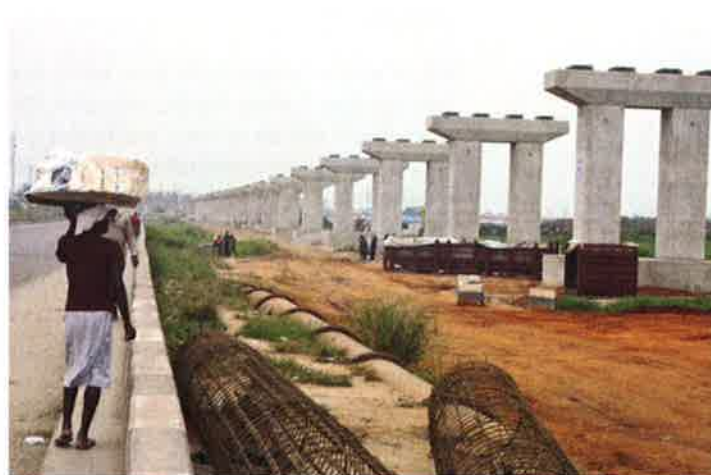
Figure 30. Lagos Light Rail Project is being done by a Chinese construction firm Chinese Civil Engineering Company Limited (CCECC), which has been operating in the country for 30 years; this project is expected to give work to 8 000 workers
